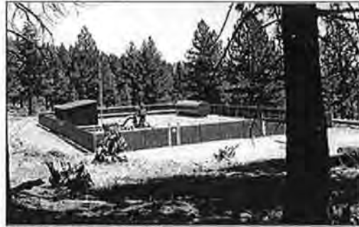
Photo of existing Geothermal well pad.
